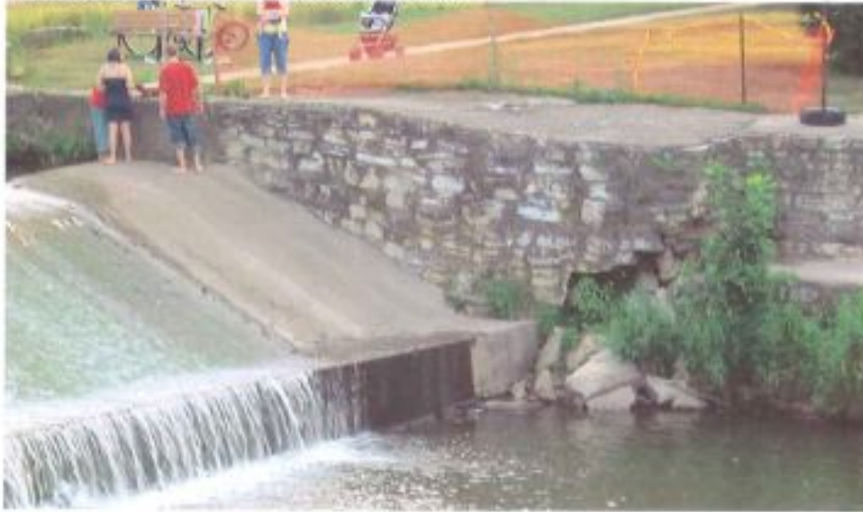
7-17-2007 PHOTO OF DAMAGED WALL
